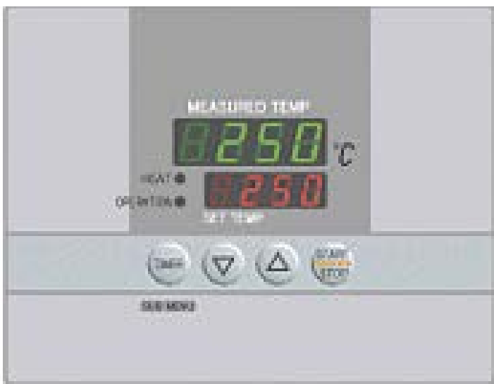
Panel de Control
